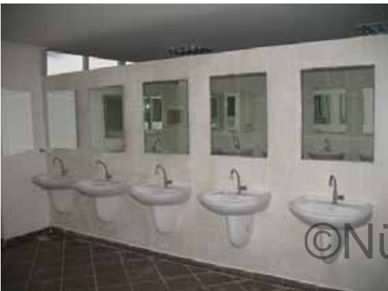
Before and after images of a bathroom in a state-run boarding school which was improved with support from the Eczacıbaşı Group
